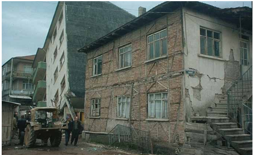
Structural failure in the concrete building in rear contrasts to the traditional building in front
